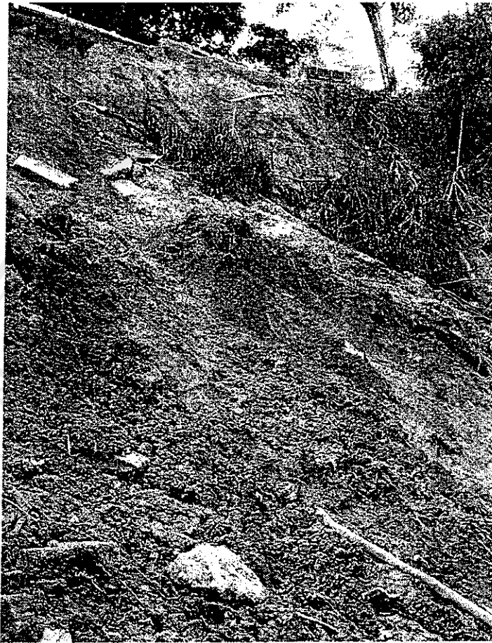
Fig. C.11 The sliding mass is still on the failure slope
