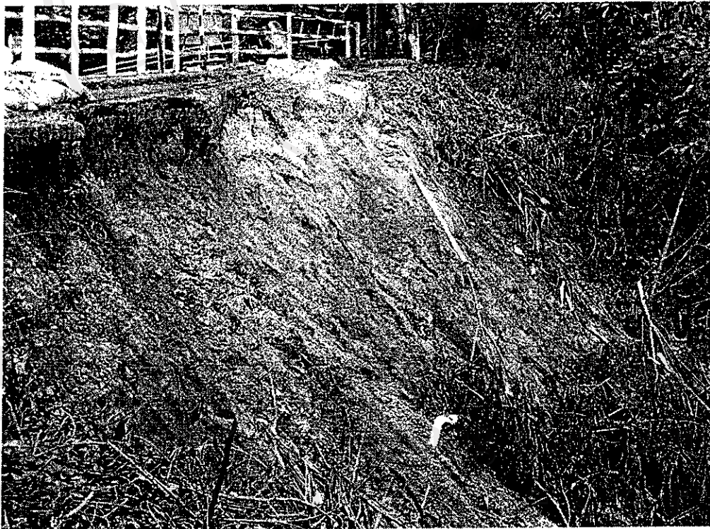
Fig. C.10 Slope failure on the right way of public highway no. 1004 at Km. 13+855.00
