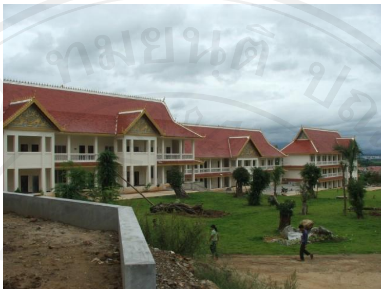
Figure 5.5: The school at Wat Luang during its construction - August 2007 (Image: Khanan Sam Sao)
