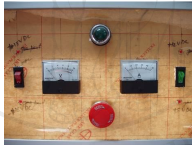
Figure 4.11 Voltmeter and Amp meter for Electronic Load
