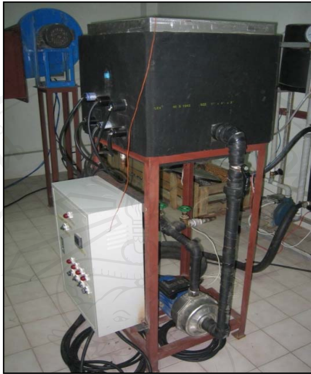
Figure 6. Heat source temperature system
