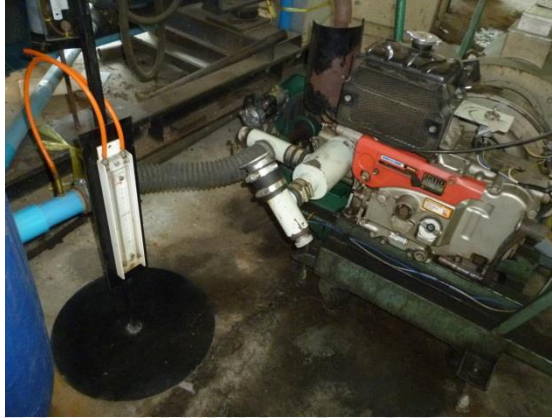
Figure 3.11 Air-gas mixer installed with small SI producer gas engine
