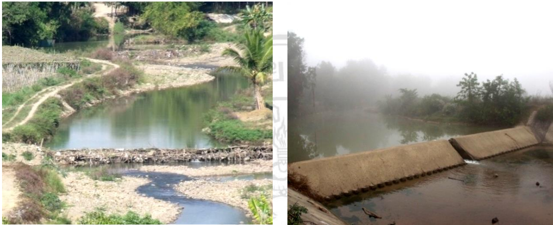
Figure 3.19 The condition of the wooden weir in 2009 (left) and the latest concrete structure in 2010 (right)
