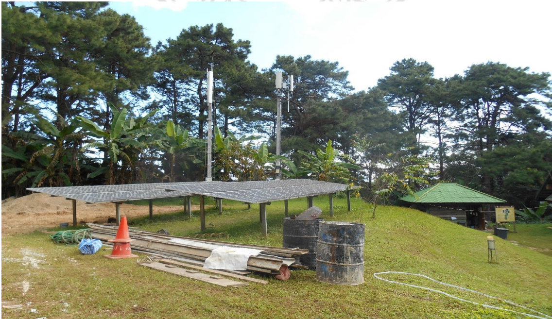
Figure 4.53 Unused solar panels at Doi Pui Campsite (Taken on 18-11-2015 by Pradip)
