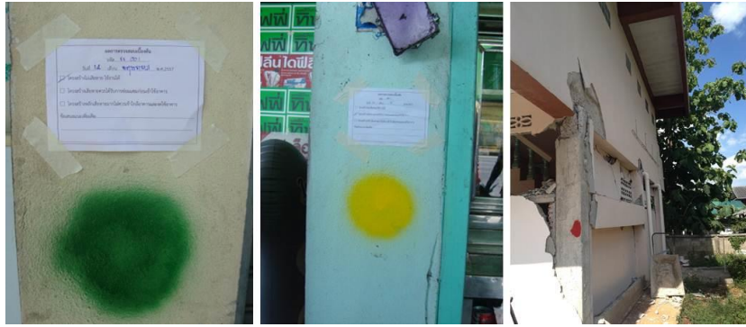
Figure 1.9 Building damage Levels (Green, Yellow, and Red paint-sign)
