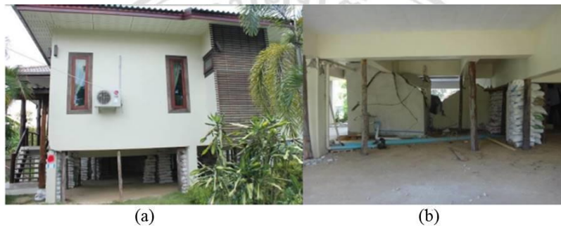
Figure 1.10 (a) An elevated one-story reinforced concrete house in Dong-Mada sub-district (b) eccentrically placed Unreinforced Masonry Bearing Walls (URM) fills and failure (Ruangrassamee, 2014)
