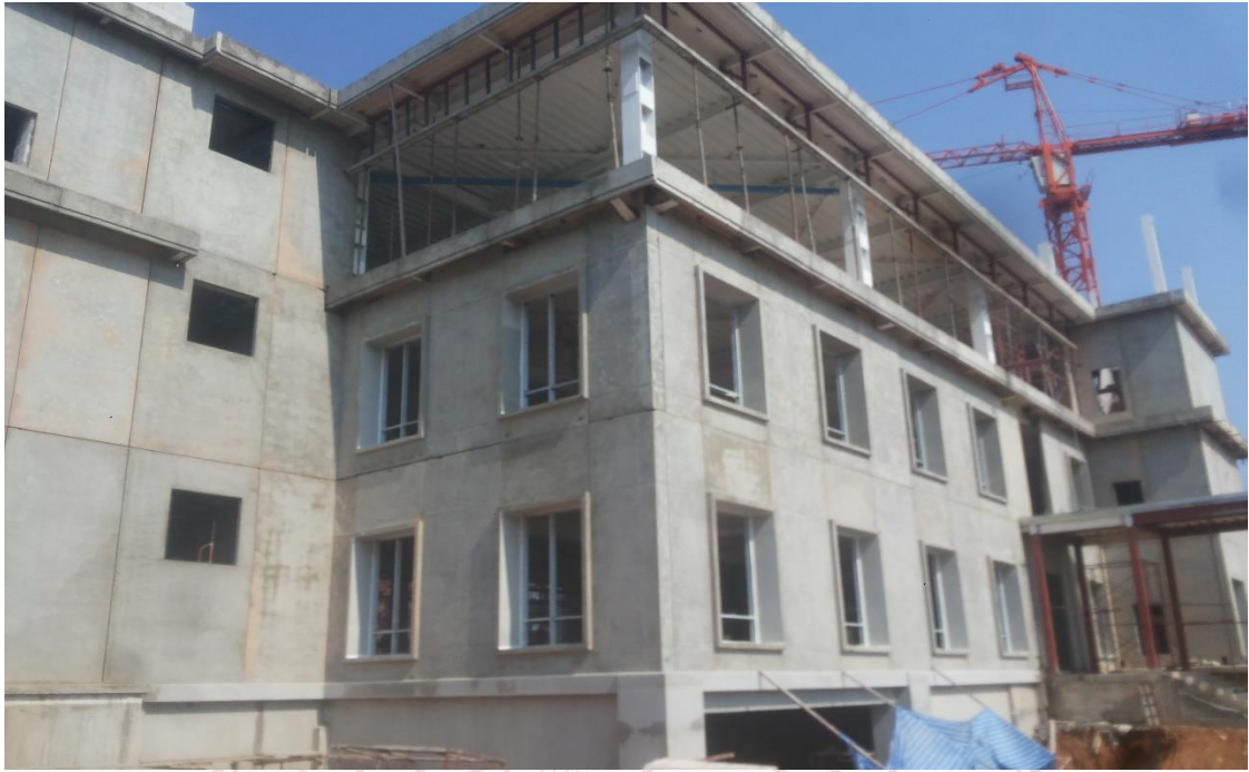
(c) Precast concrete construction for multi-story residential building Figure 1.6 Prefabricated construction in the Northern Thai region
