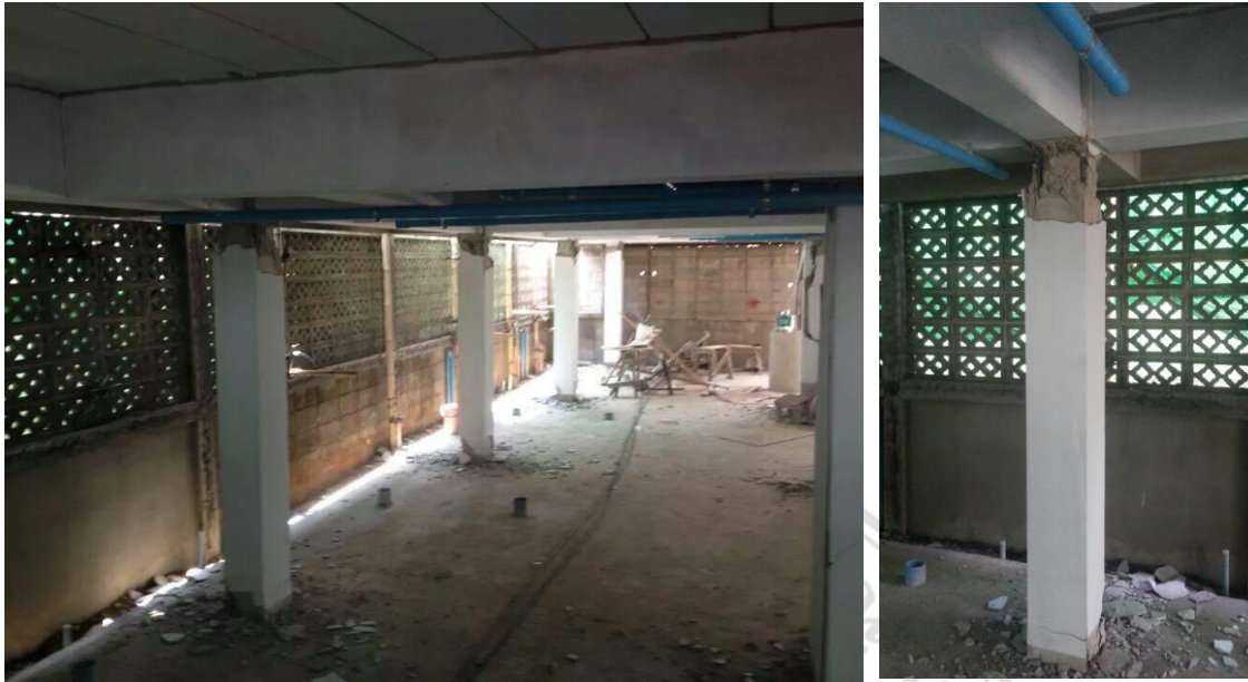
(a) Soft story collapse
