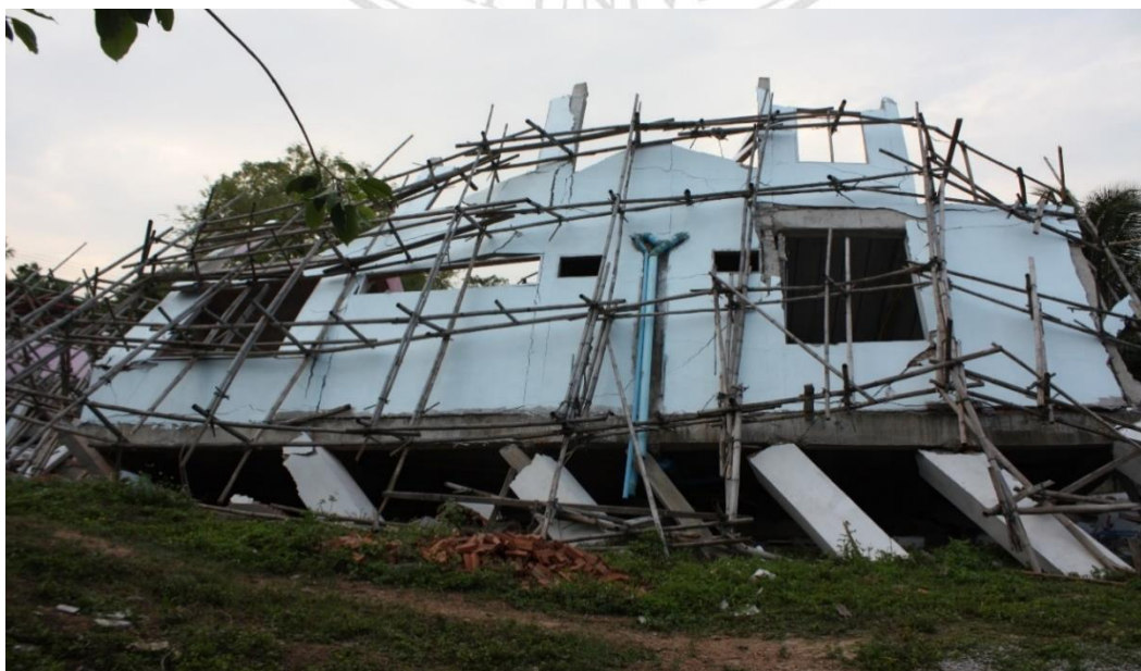
Figure 1.4 Damage from the first soft story of concrete building
