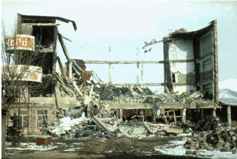
(d) Damage to Communications Building, Spitak, Armenia ( http://www.johnmartin.com/earthquakes/eqshow/647011_09.htm )
