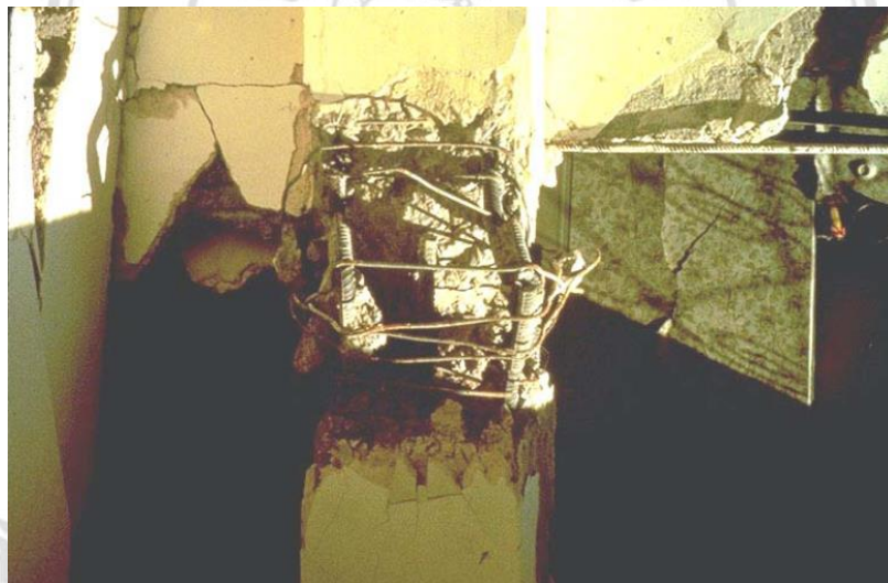
(e) Brittle failure of welded bar at the precast connection ( http://www.hellerjohnsen.com/Spitak,%20Armenia%2012-7-88.pdf )
