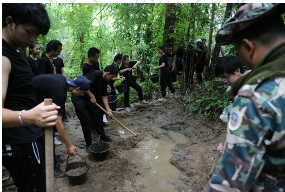
Figure 3.30 Dredging of mud around the ridge of weir to be dumped in an area around the weir, called Kaem Fai (the cheeks (sides) of weir) on 21 st August 2016
