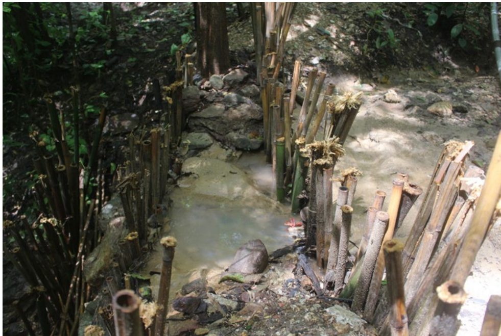
Figure 3.31 After repair, weir can retain water and slow down water current in minor stream
