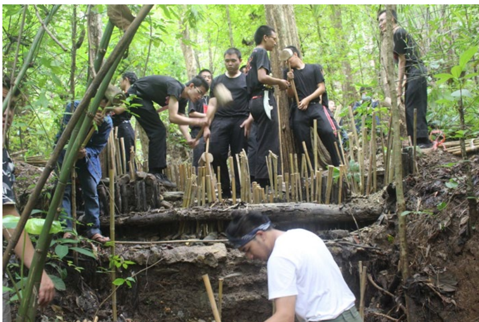
Figure 3.29 Repair of small weirs in branch stream around Mae Sa Waterfall, Mae Raem Sub-district, Mae Rim District, Chiang Mai Province, for retaining water and slowing down the water current on 21 st August 2016
