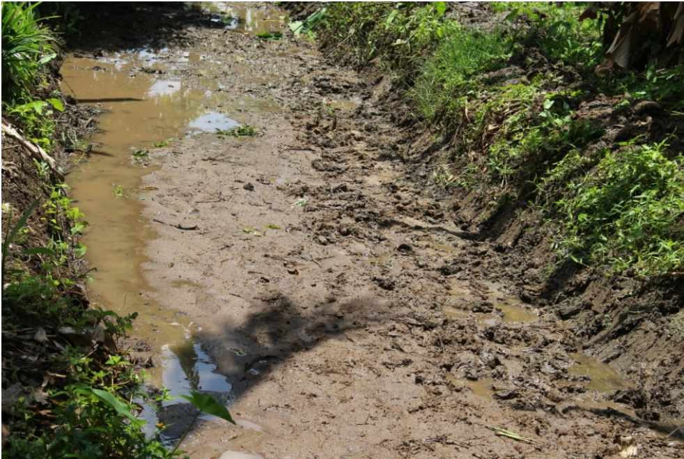
Figure 3.10 Maintenance of Ditch too Prevent Collapse
