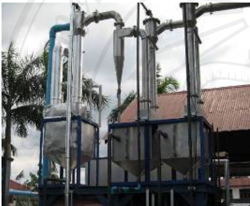
ค. Water Scrubber and Chiller Scrubber
