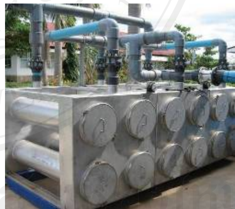
ฉ. Bag Filter Unit
