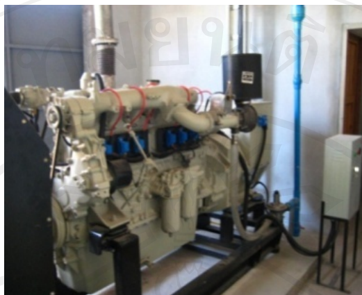
Figure 3: Generator size 100kw[7]
