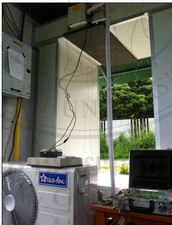
Figure 2.8 Air-conditioner installed in the testing room.
