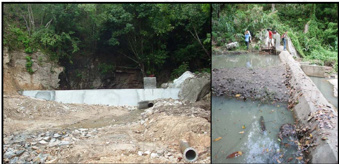
Figure 4.10 (L) The new cement weir installed on Huay Mae Hia for the Chiang Mai Night Safari's water diversion project – 2003 (source: Paki Kon Hak Chiang Mai ) (R) The onset of the weir's sedimentation problems – July 2007.
