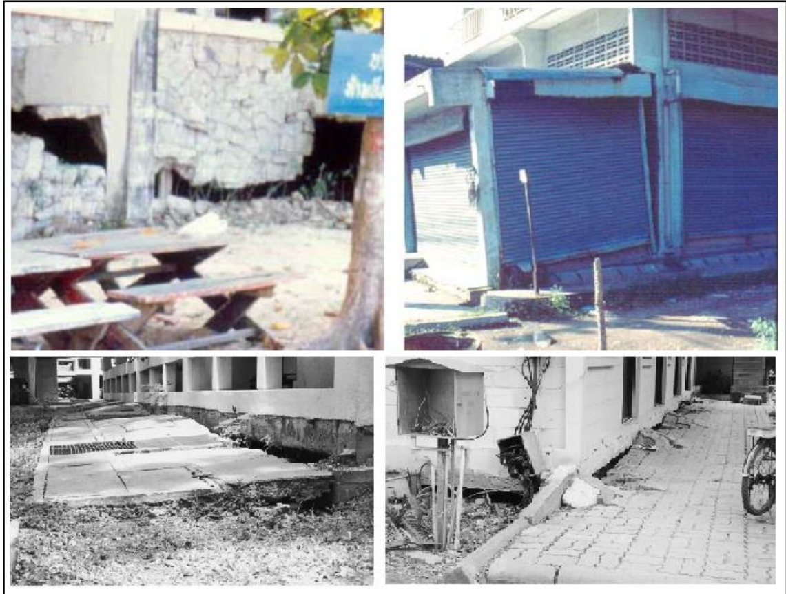
Figure 2.5 Land subsidence damage to building (after Phien-wej et al. , 2006 and 1998).
